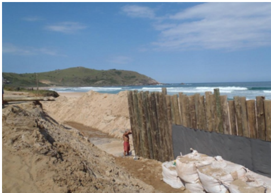
Figure 8. Building authorization for a beach vehicle path (sand) in Garopaba [SC], Brazil.
