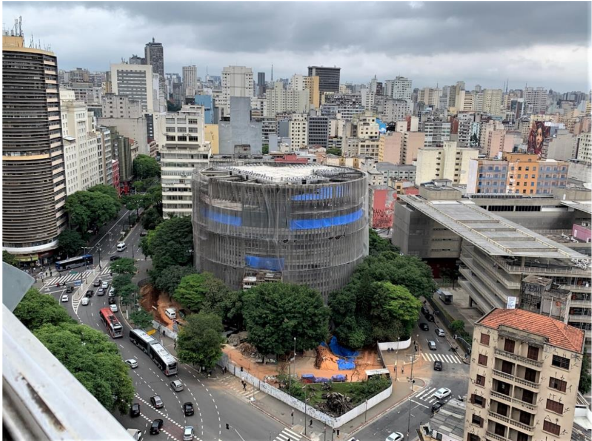
Figure 11. Alfredo building today, undergoing structural remodeling works. Please notice how fragmented the public space was when they put fences around it and the square became a private place. Photographed by the author on November 11, 2019.
