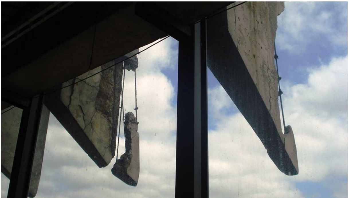
Figure 9. Alfredo Issa multistory parking garage in 2013. Notice the concrete plates dislocated from the brise soleils, Photographed by the author on February 27, 2013.
