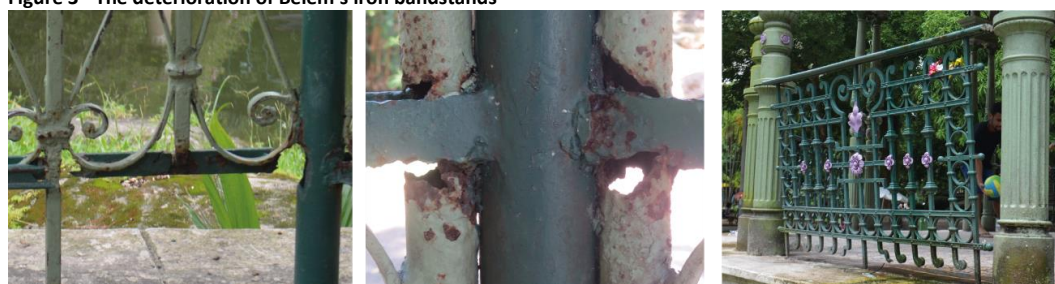
Figure 3 - The deterioration of Belém's iron bandstands
