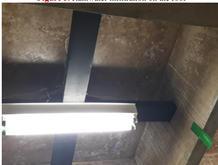
Figure 5. Rainwater infiltration on the roof
