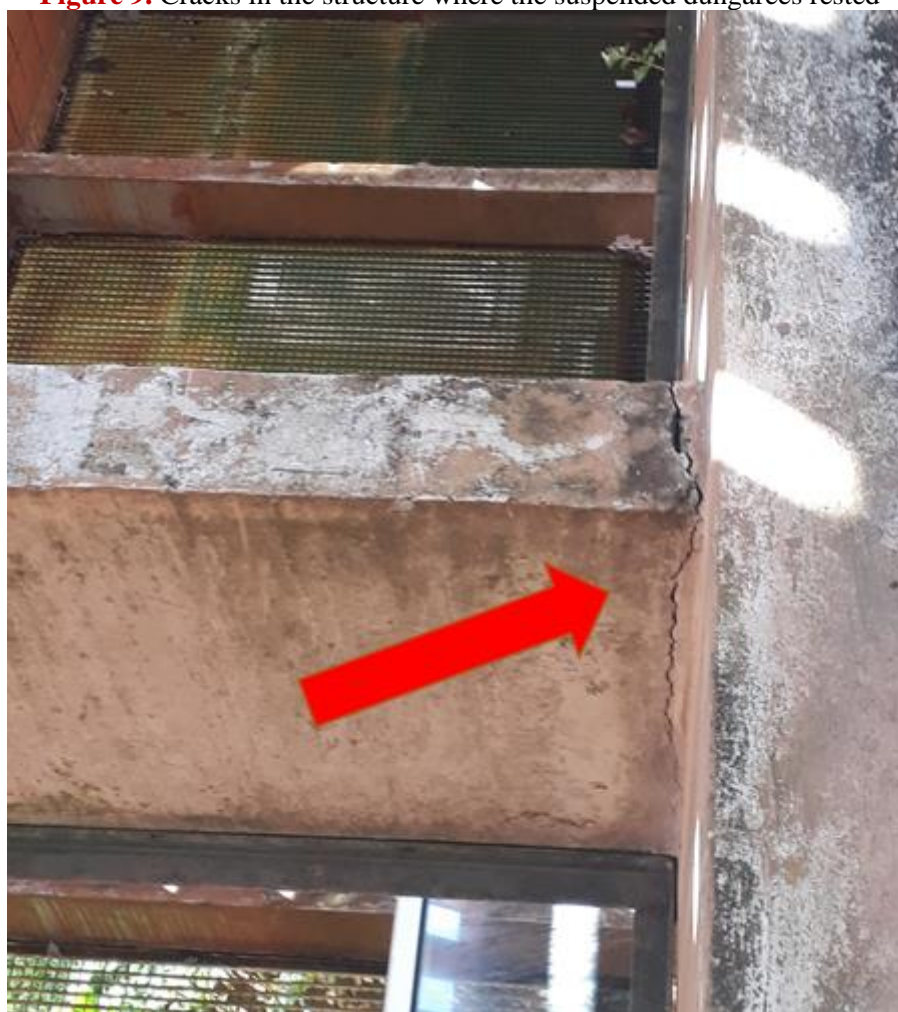
Figure 9. Cracks in the structure where the suspended dungarees rested
